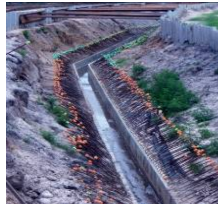
8. Bypass canal treatment trough, looking west. This system is designed to allow the treated water to flow through the trough and have the sediment fall out before the cleaned water is returned to the lake or canal.
