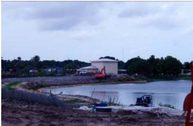
7. Bypass canal treatment trough, looking northwest. In the foreground is the treatment trough that will flow to the southeast from near the alum building in the background.
