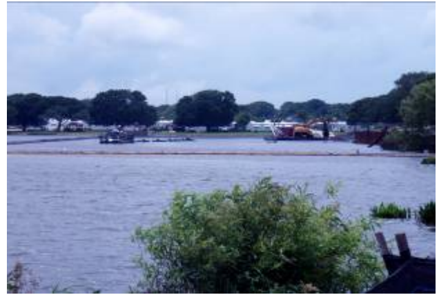
2. The in-lake alum treatment area, looking west. The suction dredge barge is on the left side of the picture. To the right, the excavator can be seen removing the dredged sediment from the temporary settling area.
