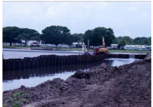
4. The in-lake alum treatment area, looking west, during the dredging process. In the foreground is the temporary sheet pile for the settling area. In the background is the excavator removing previously dredged sediment from the settling area.
