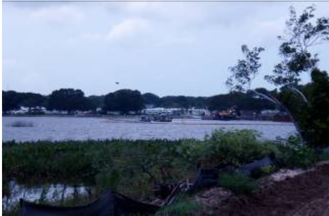
1. The in-lake alum treatment area, looking northwest. The suction dredge barge is in the center of the picture. To the right, the excavator can be seen removing the dredged sediment from the temporary settling area.
