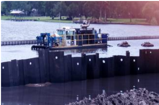
3. The in-lake alum treatment area, looking southwest. In the foreground is the temporary sediment settling area. In the background is the suction dredge barge.
