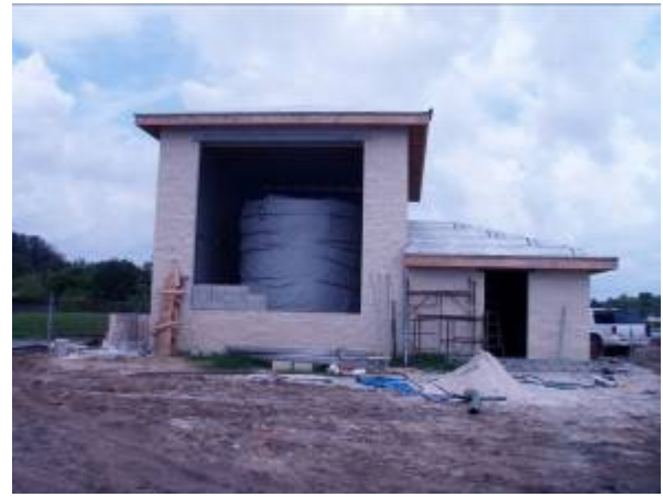
6. Looking east at the alum storage building which will provide alum to both the in-lake and bypass canal treatment systems.
