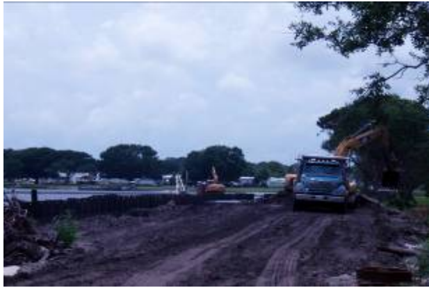
5. The in-lake alum treatment area, looking west over during the dredging process. Dredged material is being loaded onto a truck to be transported to the drying area and then later removed.
